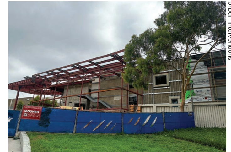
Construction continues on the $74 million first phase of San Diego High School.
