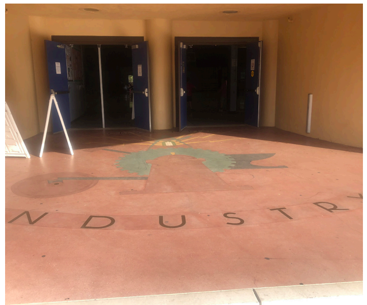
The entrance to the Municipal Gym/Palace of Electricity and Varied Industries (1935) includes this terrazzo-like treatment that will be restored in 2022 along with other artistic elements. Photo C100.
